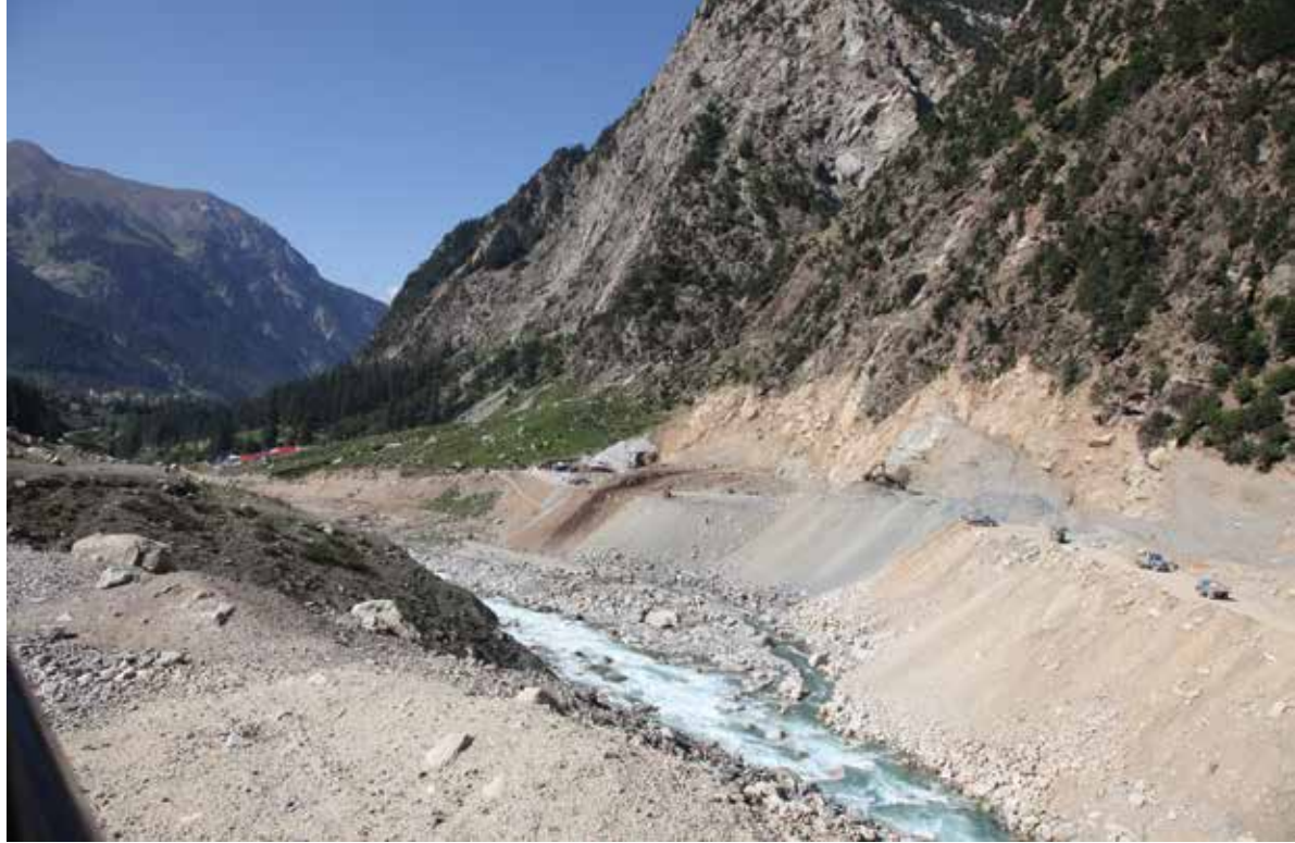
The massive earthwork of the water intake for the Chinese constructed hydropower Project in Ushu valley. 2019 .
