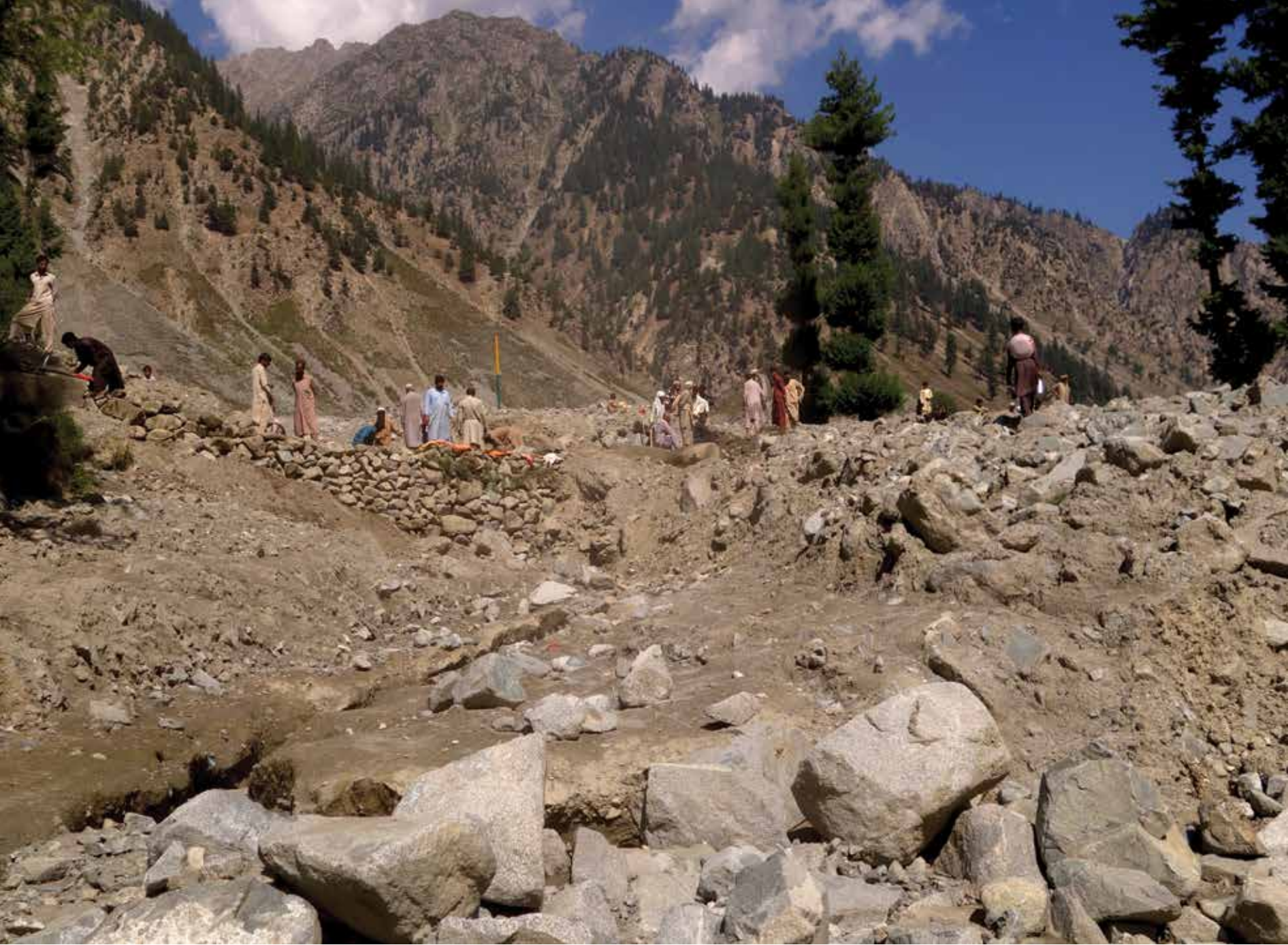
Farmers of Jabba jointly repair a water channel damaged by an avalanche during the month of August. 2019.
