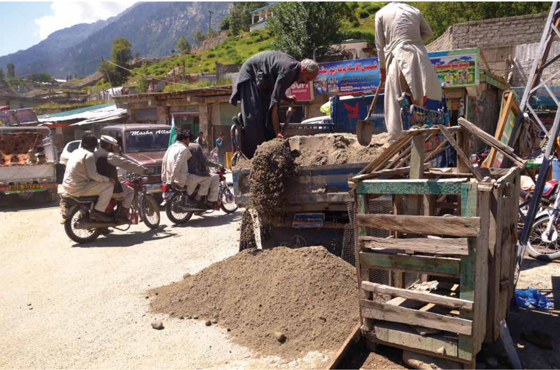
Unloading sand. The construction boom for hotels and other tourist infrastructure demands a big number of workers and specialists that Kalam cannot fulfill. In construction but also to run the hotels many people from lowland work in summer season at Kalam. 2019.
